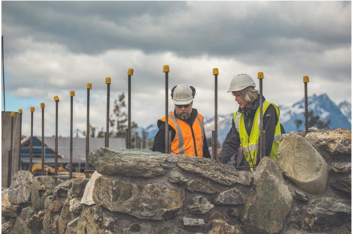
Work begins on the Scheelite Shelter with artist Dan Kelly and Jamarl Harvey, head of construction.
