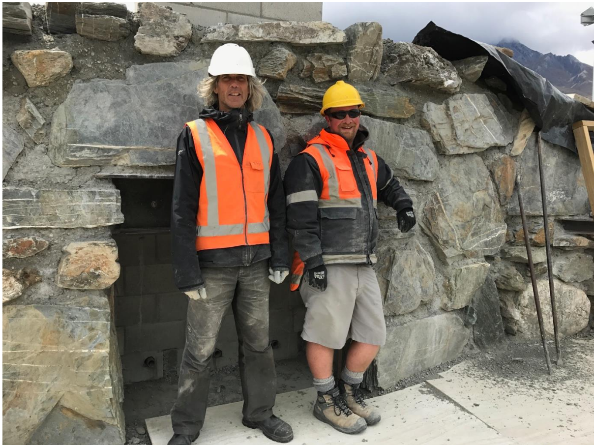
Dan Kelly and John Golden at work building the Scheelite Shelter and Cookhouse at Camp Glenorchy.
